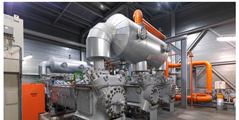
H 2 pipeline injection, Type: 6B2AC, Botlek Netherlands
