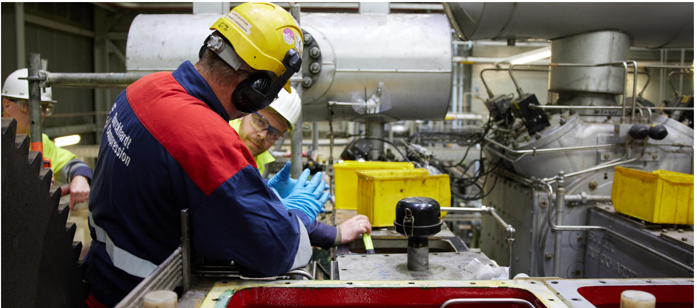
Careful inspection of compressor components, including sealing systems, is essential to identifying leaks
