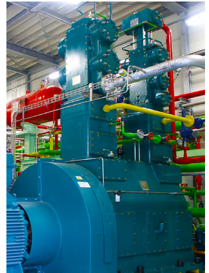
One of the two high-pressure hydrogen compressors — faithfully running since 2001.
