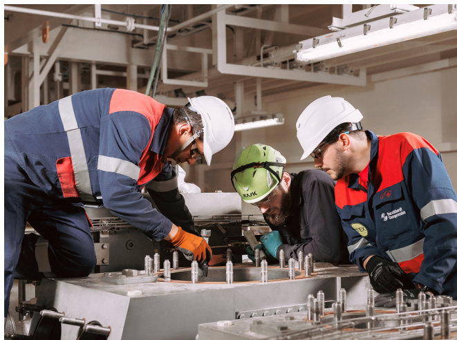
Coordinated compressor maintenance in dry-dock is crucial for long-term efficiency and reliability
