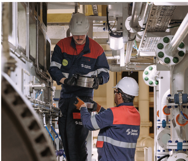
Burckhardt Compression can deploy experienced personnel and their equipment to support planned maintenance in shipyards, ports or at sea
