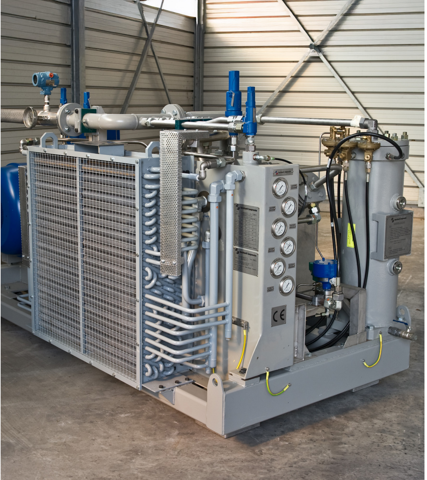
CU compressor meeting high safety standards in a hydrogen bottling plant
