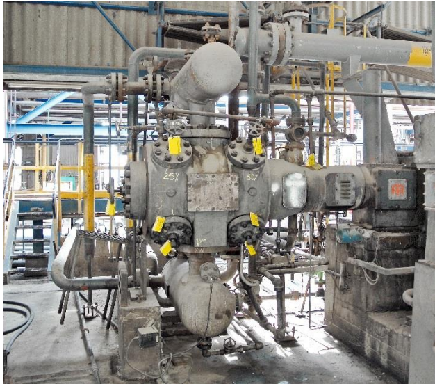
Original cylinder with indicated leakages
