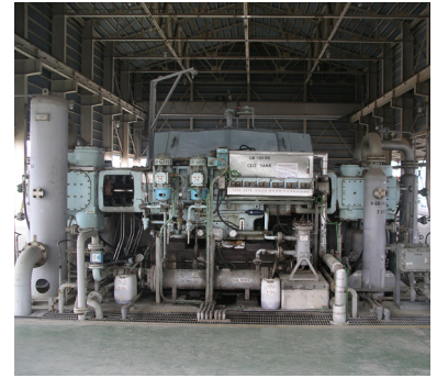
Process Gas Compressor as a Booster/ Primary compressor before the revamp
