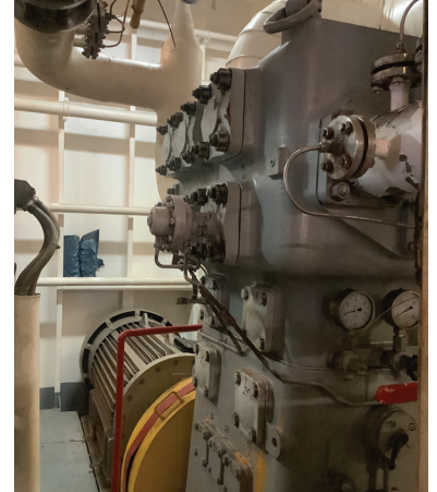
New cylinder was needed to restore operation
