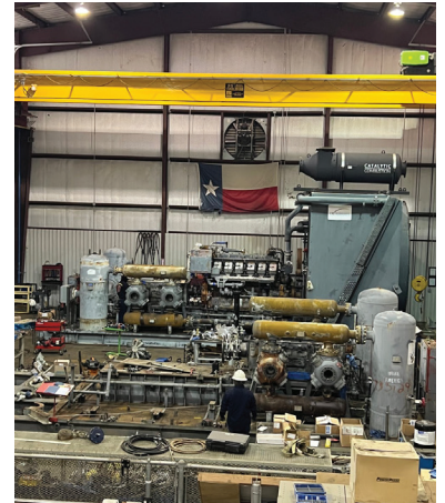
Compressor packages at Kilgore Service Center
