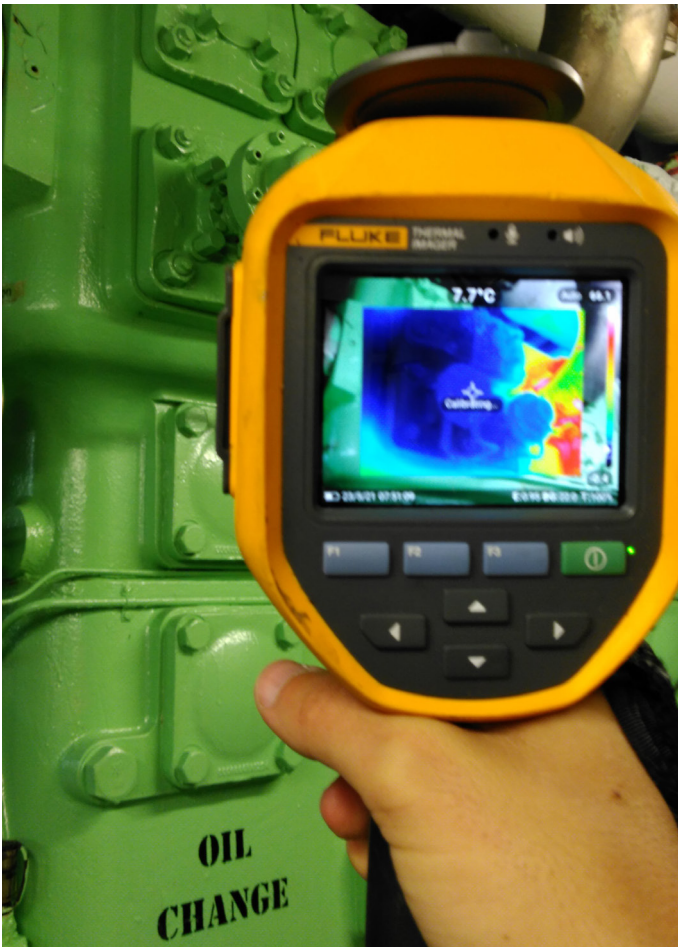
Image 4: Thermal imaging is one of the methods of identifying gas leakage, which can lead to reduced efficiency and reliability in a compressor
