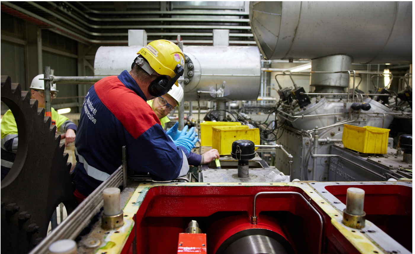
Image 1: Careful inspection of compressor components, including sealing systems, is essential to identifying leaks
