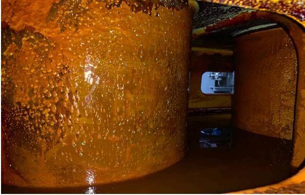
Image 2: Corrosion caused to cylinder water chamber due to an incorrect glycol mixture.
